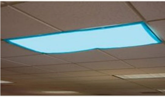
Diffuser for fluorescent Lights
